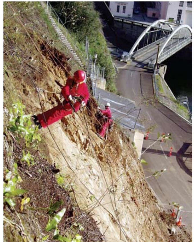
TOP LEFT. Tree felling above State Highway Two Wairoa. TOP RIGHT. Devegetation, Whakamaru. BOTTOM. Slope remediation, Karapiro.
